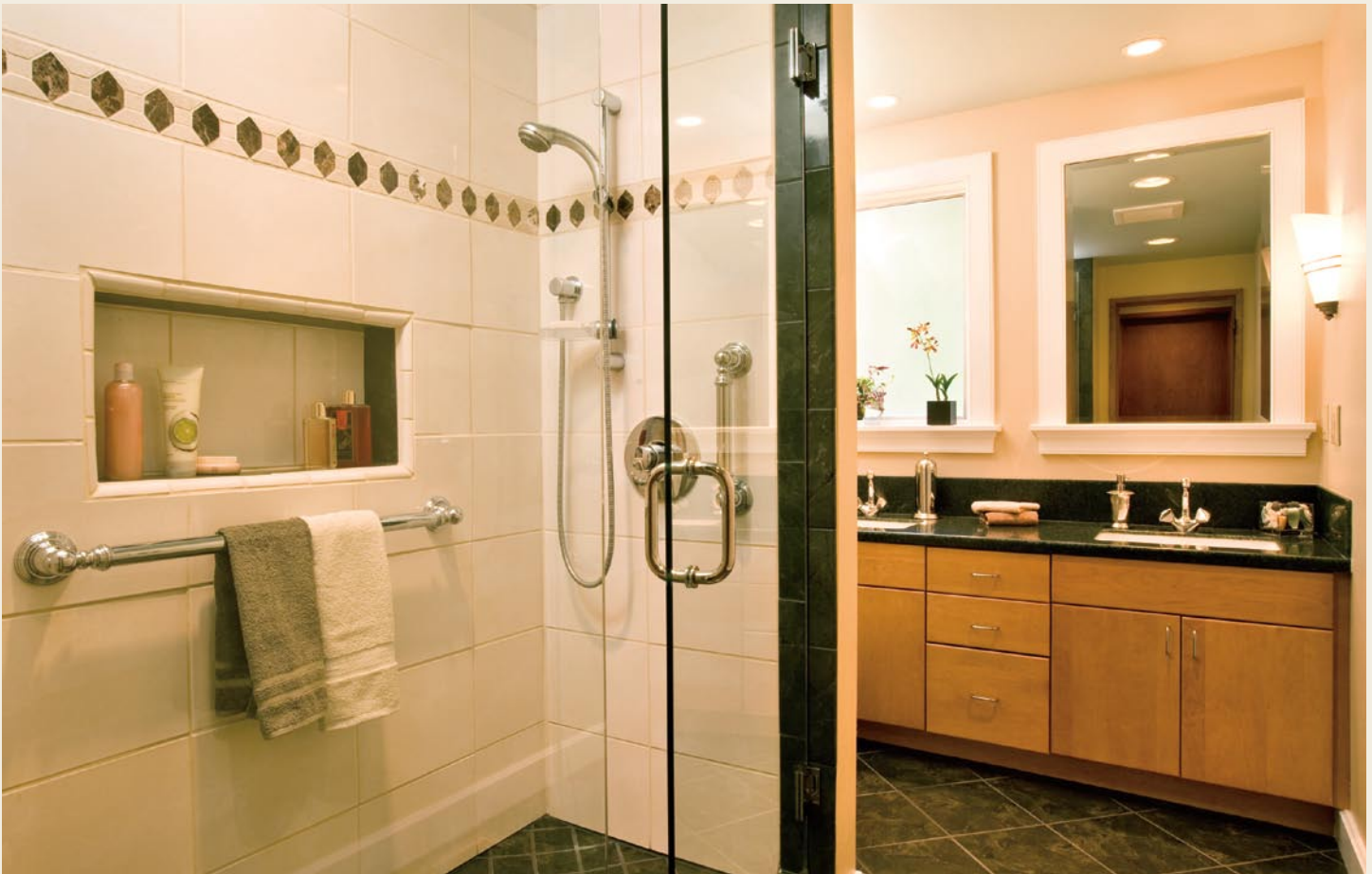
Repeat client Pam Cross will not have to remodel her bathroom again after Irons Brothers Construction redesigned her old bath using universal design standards, including replacing a bathtub with a new tiled-in shower. © Scott Chytil Photography.
